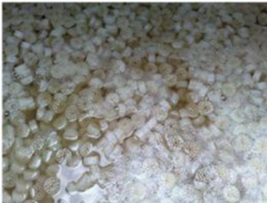
MBBR media without aeration
