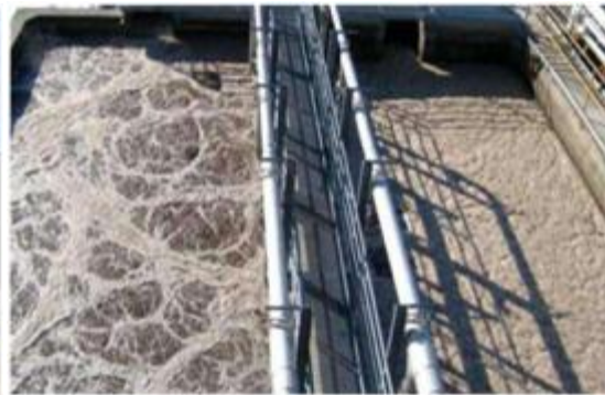
MBBR media in sewage treatment plant
