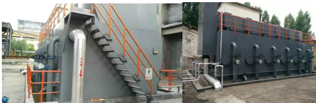
Electroplating plant in Sichuan, China
